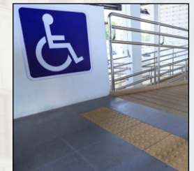
Disabled Persons' Ramp
